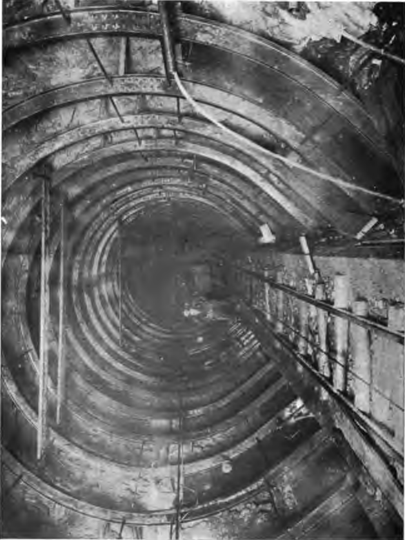
PLATE 95. —Rondout Siphon. Steel Shell in very Wet Ground North of Shaft 4. Invert in place. Plates of interlining packed with broken stone to conduct water to drain in invert. Many springs were led directly through pipes to facilitate grouting.
